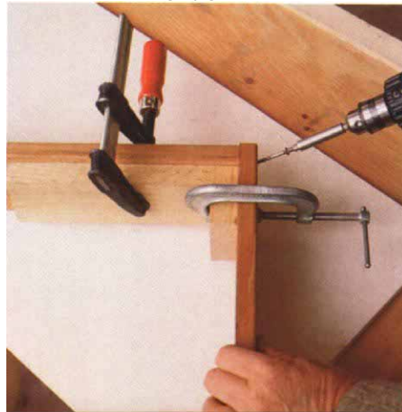
Two clamps. A quick-action clamp on the left and a C-clamp on the right secure a jamb extension to a 90° angle jig.
